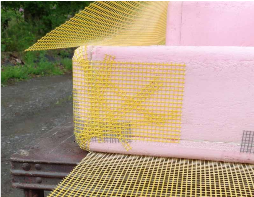
Top: Cut and fold down narrow fingers of mesh at each of corners. Bottom: Fold the wide flaps of mesh down over the fingers.
