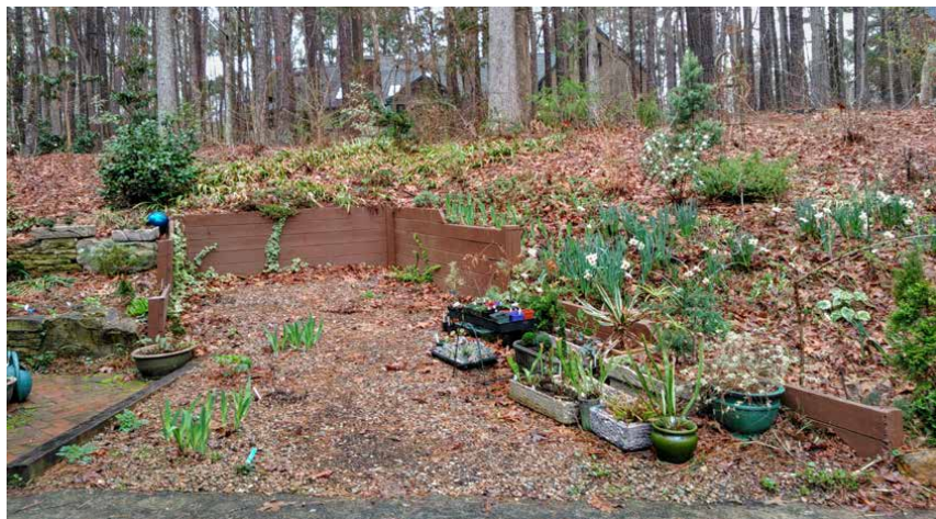
Above: The space before constructing the crevice garden. Opposite: The finished, planted, garden.
